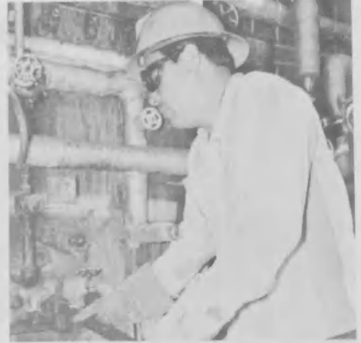
Jacinto Croeze wears asbestos gloves to pull out a burner gun from boiler at the Edeleanu Plant.
